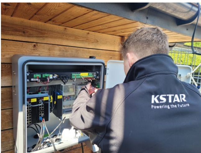
Installers are debugging the product
